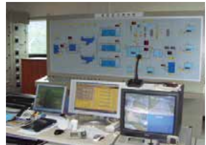
<Remote controlled automated water treatment plant>
