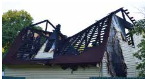
Types of damage caused by direct lightning strikes: buildings, lives, etc.
