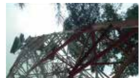
Thailand Navy Satellite Station
