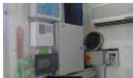
Airports Authority of India Glide Path
