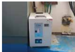
▲ Water purification plant automation control system
