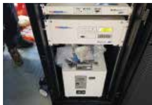
▲ TRS Mobile Relay Station
