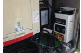
▲ Water purification plant flow meter
