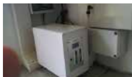
Malaysia Airforce Localizer station
