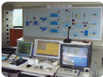
<Water Plant control>
