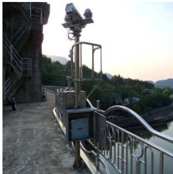
Dam Discharge monitoring CCTV
