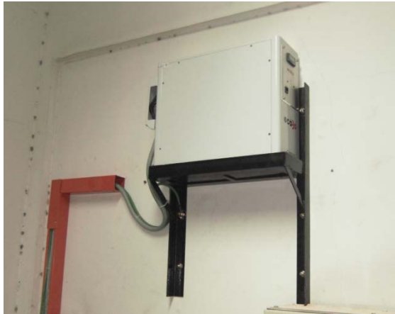
<eca3G-LM > installation : parallel connection at UPS
