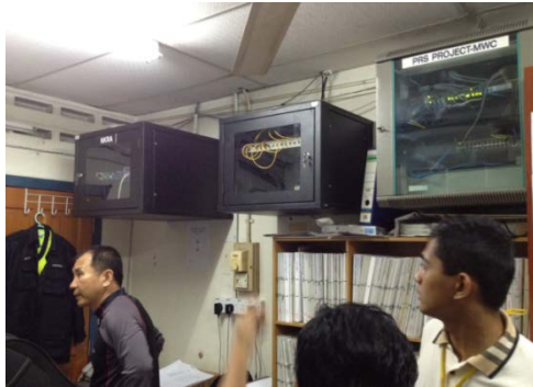
PRS Cabinet without Grounding
