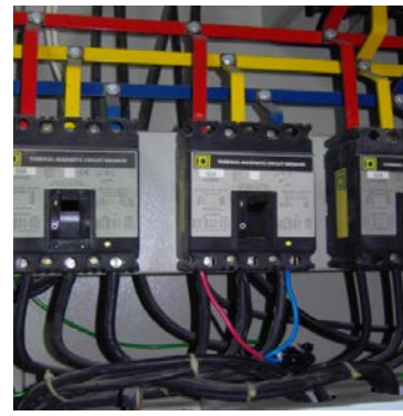
<eca3G> cabling to 3 live lines
