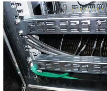
Improve Rack Bonding
