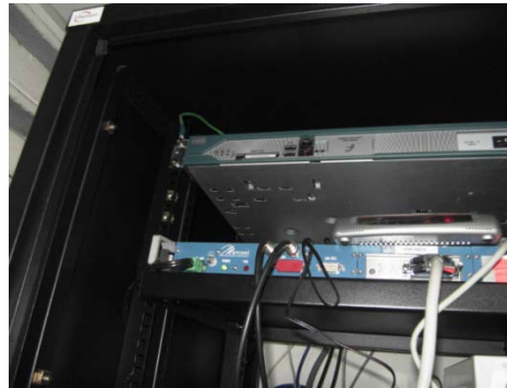
Grounding improvement for equipment
