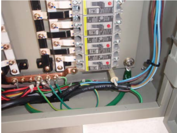
Grounding bar at Southern airway shelter
