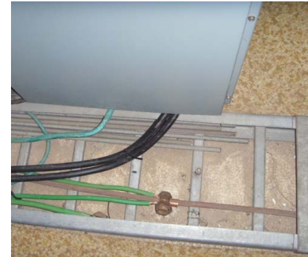
Main Ground bonding
