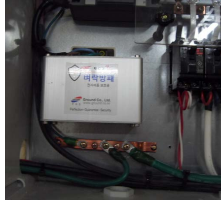
<eca3G LP> Installation
