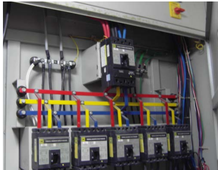
Main DB ( 3 phase, 4 wire )
