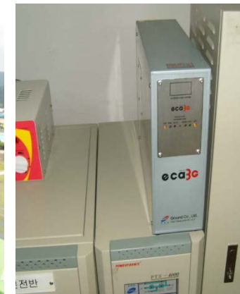
Dam control system
