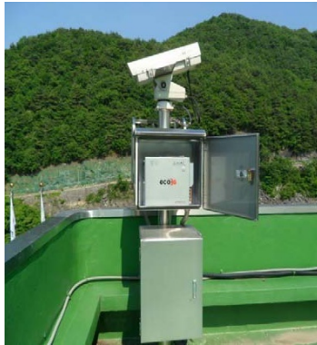
Building Roof gate CCTV
