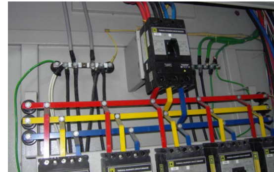
<eca3G> cabling to Neutral Terminal & Ground Terminal
