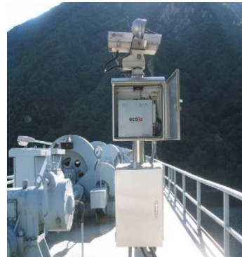
Dam upstream CCTV
