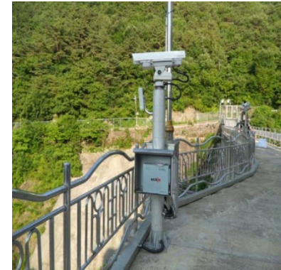
Downstream monitoring CCTV
