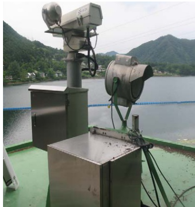
Bridge Road guard CCTV
