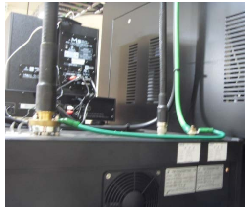
Rack, Transmission line bonding
