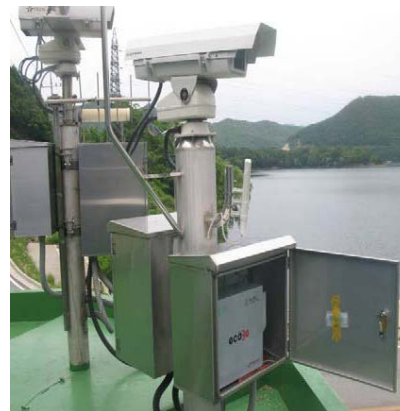
Dam downstream CCTV
