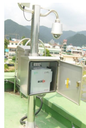
Pump room Roof CCTV
