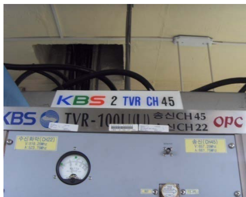
Transmission system Rack
