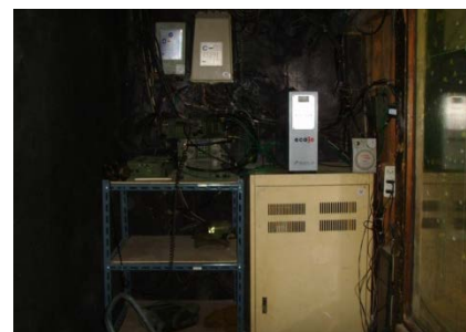
Communication system bonding
