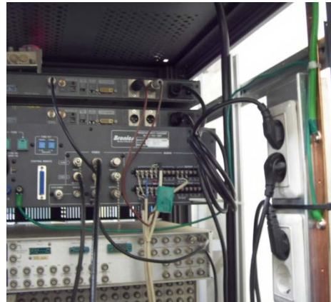
Equipment, Rack bonding
