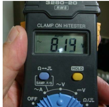
N-G potential before installation
