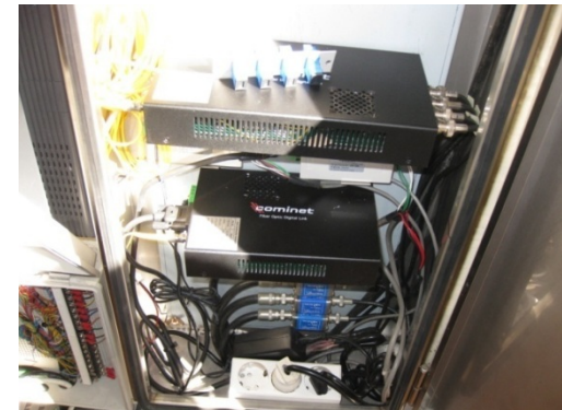
Shield of signal cable – G - potential 19.5 V (not grounded)
