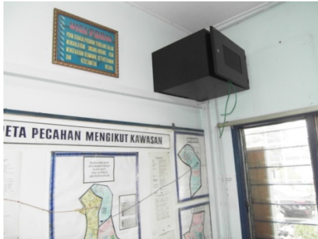
Grounding connection to PRS cabinet to <eca3G>
