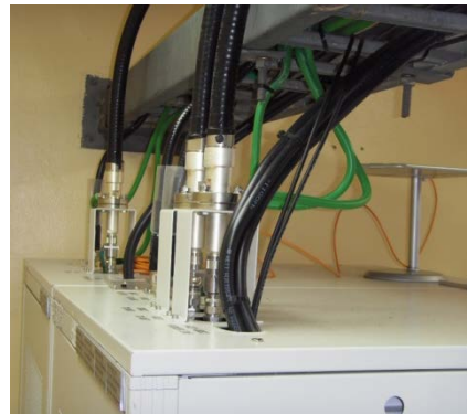
Aerial cable bonding
