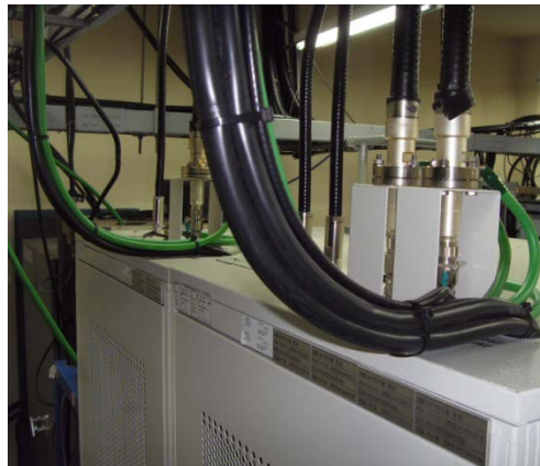
Aerial cable bonding
