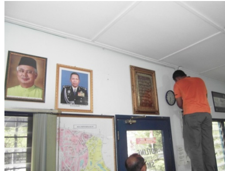
Grounding cabling : bonding improvement
