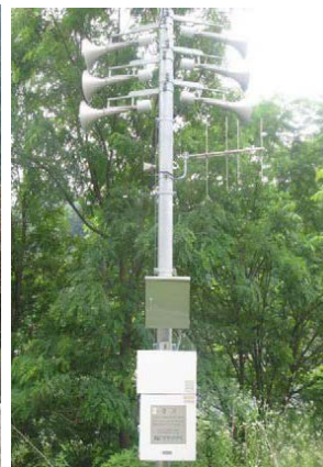
Discharge Alarm system
