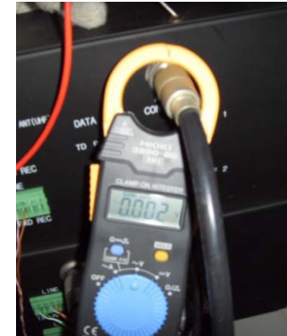
Repeater Rack equip- potential
