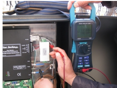
SPD & G terminal of Detector / Alarm - potential 12.23 V
