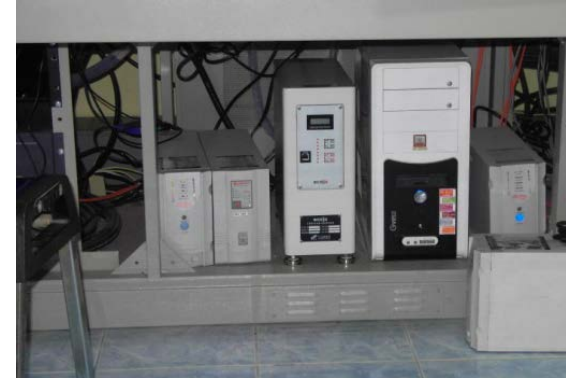
<eca3G-LM > positioning to protect three UPS and Monitoring systems
