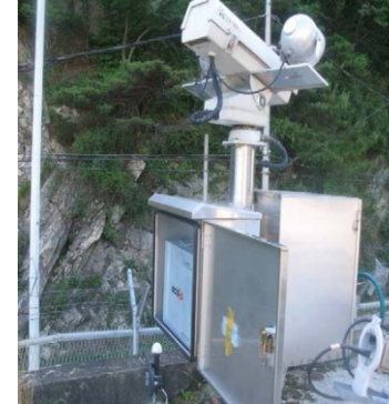
Bridge Road CCTV
